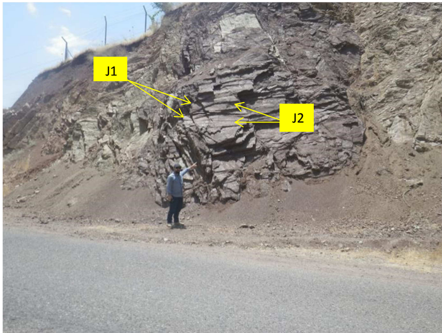
Figure11: site No.23 showing the detached blocks due to differential erosion
