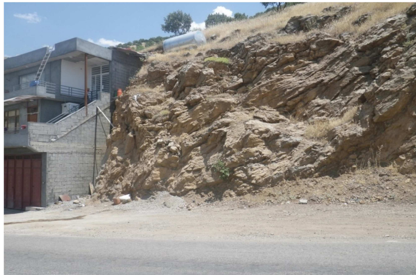
Figure 9b: lateral view of the site No.22 showing wedge sliding
